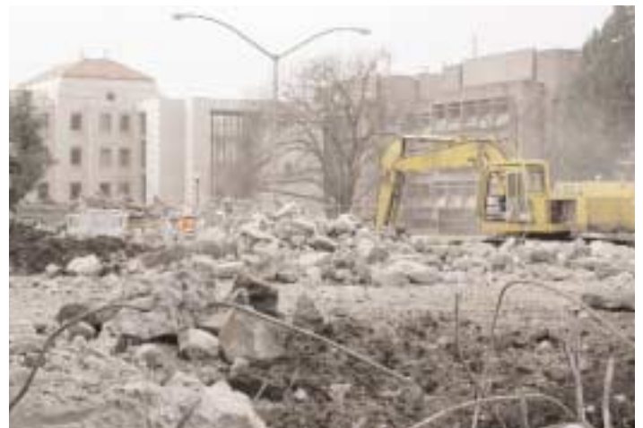
The Life Sciences Addition and Briggs Hall rise above the rubble on the site of the future Sciences Laboratory Building
